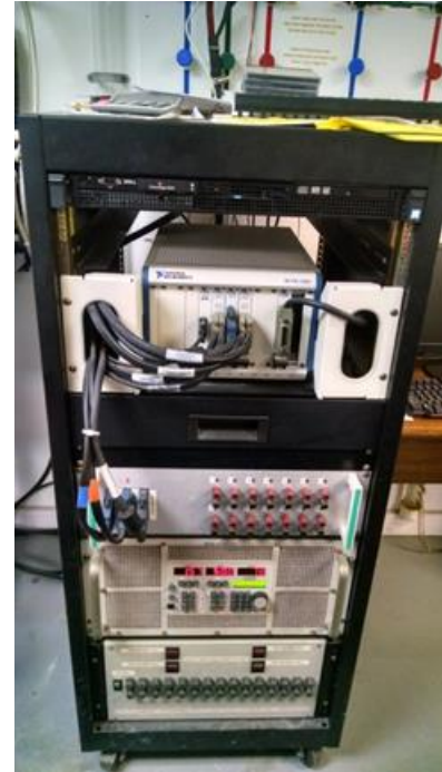
Figure 5. The power supply (second from the bottom) reads 50.0 A
